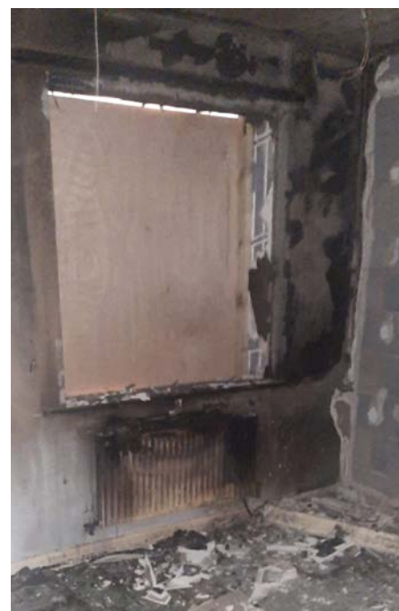
Fire damage in Kirsty's home
